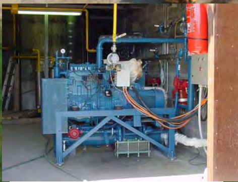
Combined heat and power
