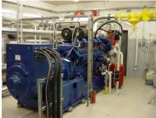
Figure 4.8.3 A 16 cylinder 35 litre gas engine used to produce electricity in Alvik
