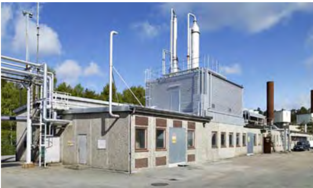
Figure 4.6.1 The upgrading plant at Arendal, Gothenburg
