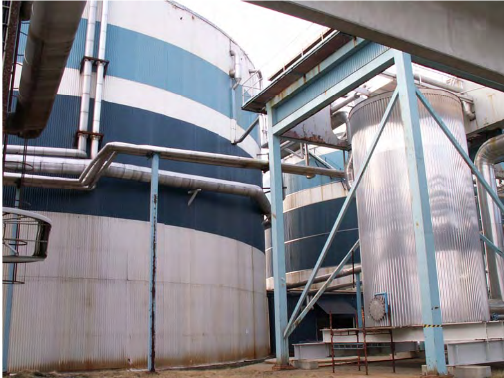
Figure 5.11.1 The biogas plant at Domsjö. The blue and white tanks are anaerobic digesters and the polished steel container is a de-gassing tank.
