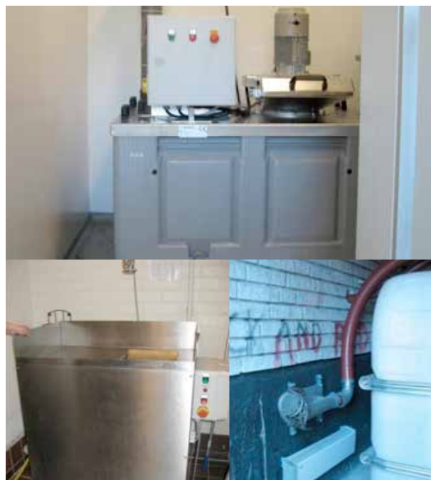
Figure 15: A grinder and a tank connected device (left). A simpler solution, with a grinder in the kitchen connected to the waste tank placed in a garbage room (right). (Source: Stockholm stad)
