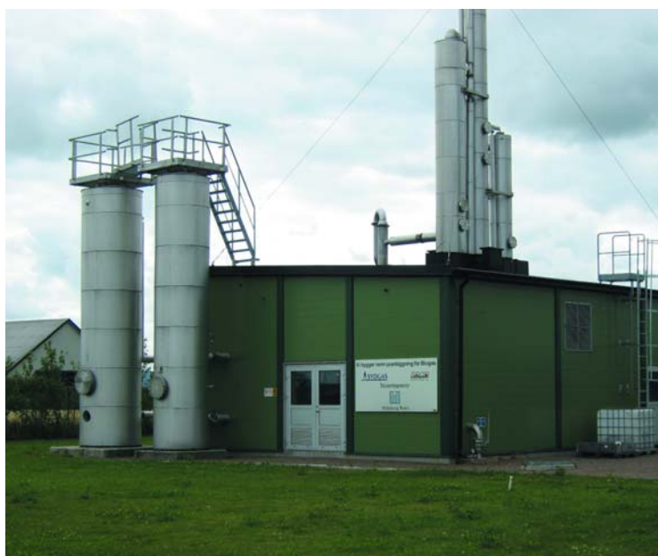
Biogas from the Laholm plant is upgraded to natural gas quality in a Selexol plant with a capacity of 500 m 3 /h
