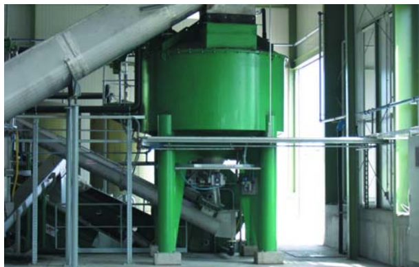
Fig. 3: Pulper unit optionally used for waste liquefaction resp. contaminant removal
