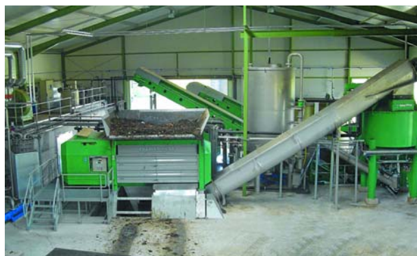
Fig. 4: Overview of the mechanical waste pre-treatment part of the biogas plant Marchfeld
